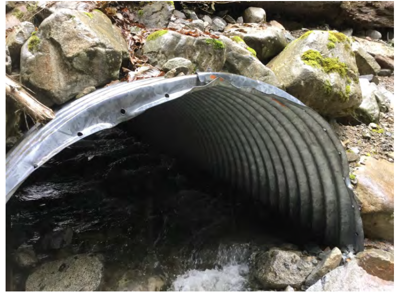
Some damage to outlet of culvert
